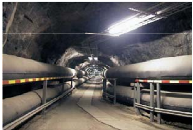
Figure 4, Tunnels utility corridors "utilidor"
